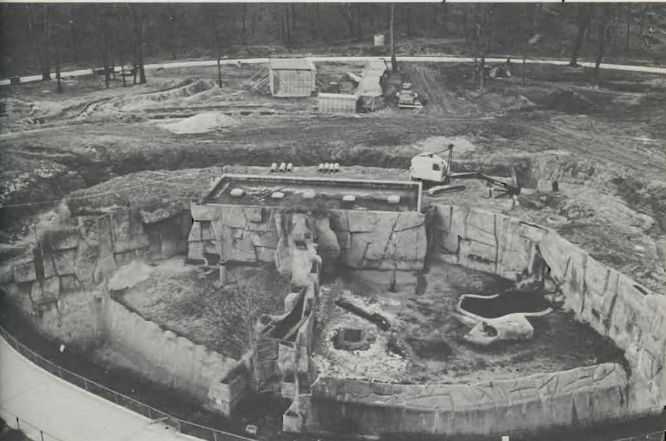
Construction site for Cleveland Zoo's new moated bear grottos and hoofed animal complex as seen from the Fulton Road Bridge. Immediately behind the Lion and Tiger Veldt is excavation for the new bear moats. Moats for the hoofed animal paddocks may be seen in the left and center backgrounds.
