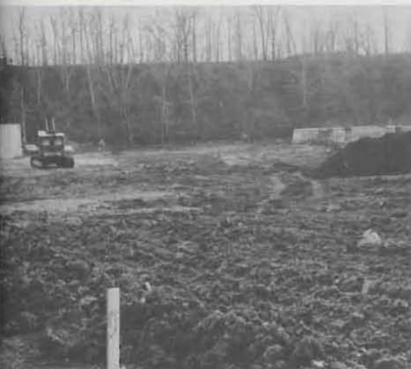
At the construction site looking in a southeasterly direction, hoofed animal moat is seen in right background. Link-Belt shovel operates in area where bear moats will be located.
